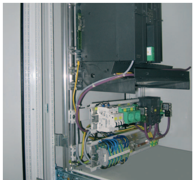
LSC-BRACKET system in the programming cabinet
